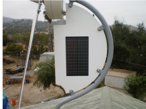
View of Solar Panel
