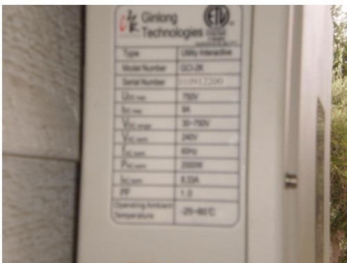
Nameplate on Inverter
