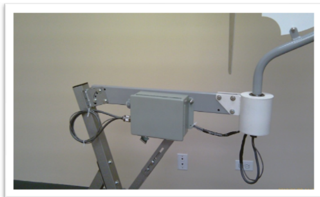
Image 1 – Rectifier installed on Frame Shaft
